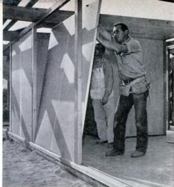
Carpenters raise pair of exterior wall panels into place. Interior space saved by thin walls amounts to 150 square feet
